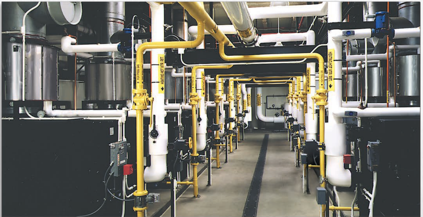
College Campus , Long Beach, California (10) EM Series boiler economizers preheating hot water return loops.
