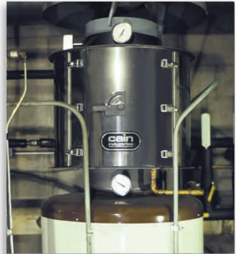
Condominium Complex , Milwaukee, Wisconsin EM Series economizer, on top a domestic hot-water heater, preheating municipal water.
